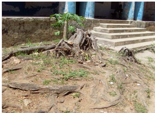
ROOTS UNDER THE BUILDING
