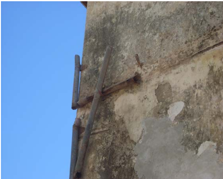
DELAPIDATED DRAINAGE SYSTEM
