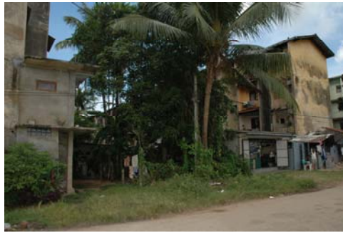
Violations of building regulations by extensions & encroachments.
