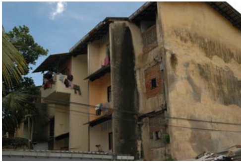
Unsafe extension in the 3rd floor
