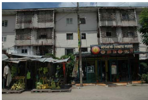
1st floor house has been extended & converted for commercial activities without considering natural lighting & ventilation.
