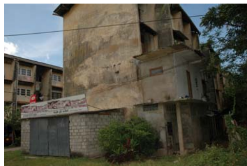
1st floor house has been extended. Ground floor has been encroached to build a garage.
