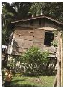
Figure 7b; Lack of bracing caused damage after earthquake
