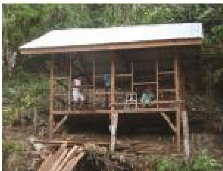
Figure 7a; Lack of heavy foundation
