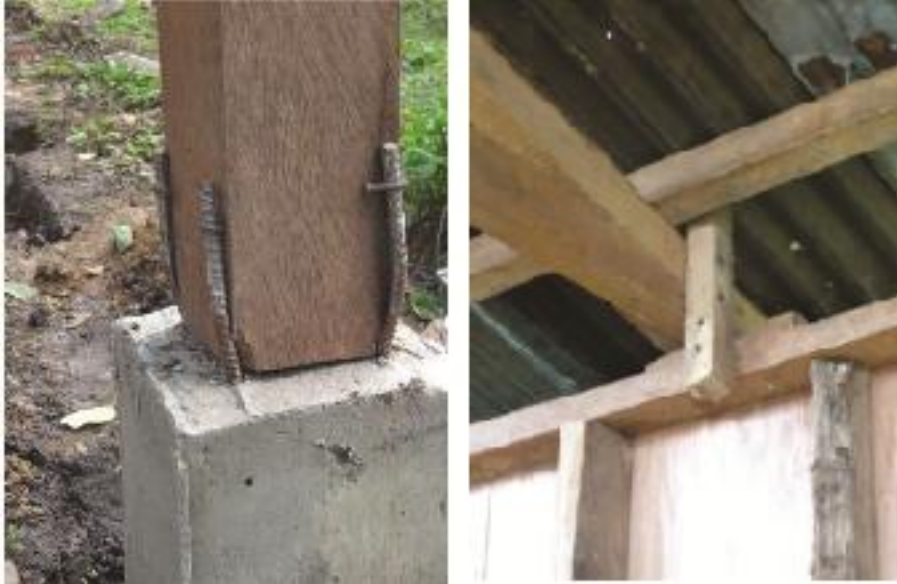
Figure 10; Examples of poor connections with only nails found in Bohol
