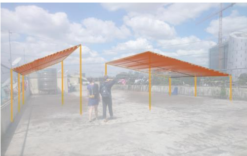
Illustration 12 Putting some shading devices will increase the use of a place previous "dead".
