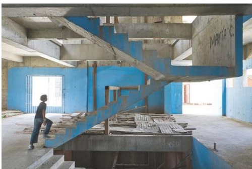
Figure 8: Staircase without railings posing a danger to the dwellers' safety (Schwartz, 2014)
