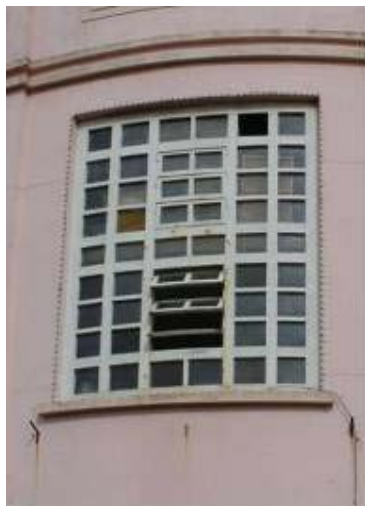
Figure 21: Window detail with missing glass
