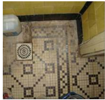
Figure 24: Bad condition of internal hydraulic bricks (2007)
