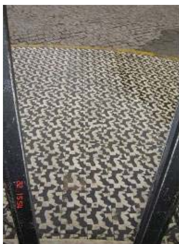
Figure 22: External hydraulic brick flooring is dirty, spent and presenting many missing tiles
