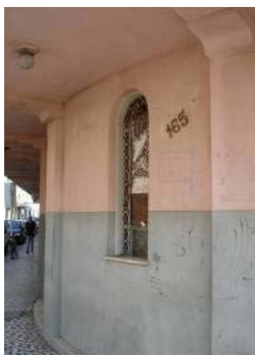
Figure 23: View of exterior wall and window with missing steel railings
