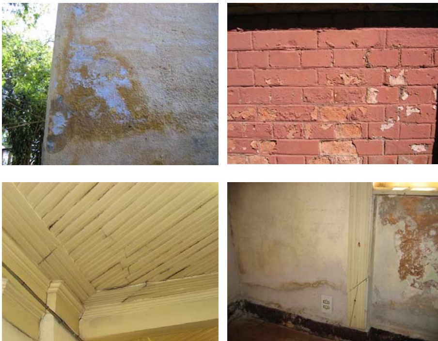
Figure 15-18: Damages: infiltrations, leakage, humidity, sunlight effects, inadequate plastering.
