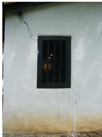
Figure 9: Cracks on the south-eastern wall.2007 Photo: Aline Carvalho
