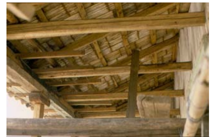
Figures 20: Similar system than described in previous figure, this time applied in a Galleria. The eaves are cantilevered in both directions and clay tile is supported in a reed mat.
