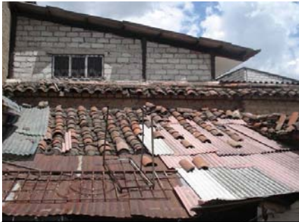
Figures 22: This kind of destroyed panorama is more and more often. Tiles become a pathetic vestige among new materials chaotically used.
