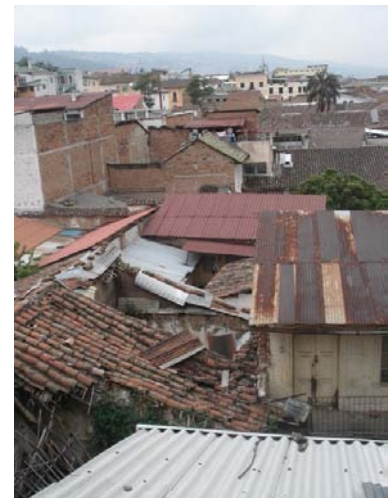
Figures 30: Multiples roof damages: replacement of coverings by metal or fibrocement sheets, collapse of traditional clay tile roofs.
