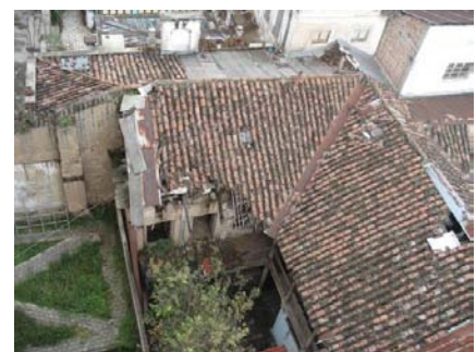
Figures 21: Alarming levels of deterioration and introduction of modern materials to patch tiles dissemination.
