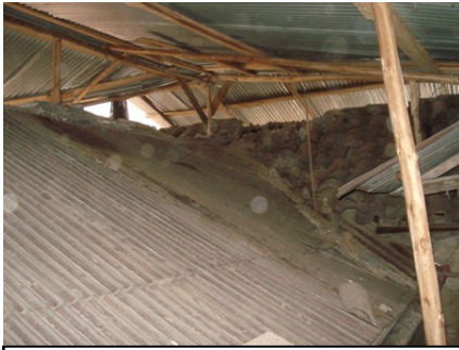
Figures 27: Roof intervention under temporary zinc cover. Note the utilization of fibrocement sheet as waterproofing layer.
