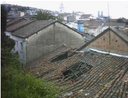
Figures 24: Partial Collapse of roof due to clay sliding, progressive infiltrations and consequent lost of structural integrity. No subsidy or specific intervention is implemented by the Municipality to address this common case of alarming affection.
