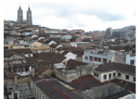
Figures 13: “Roofscape” from Manabí Street towards the Basilica. Note roof deterioration in first plane of the image.
