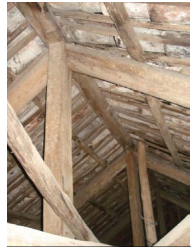
Figures 29: Roof at risk. See the trusses knot system and tiling battens. Dots are indicating xylophage's activity.
