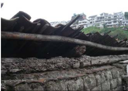
Figures 23: Ridge, “chaguarquero”, wooden chords on adobe walls. Typical damages and deteriorations due to weather exposure and lack of adequate architectural details.
