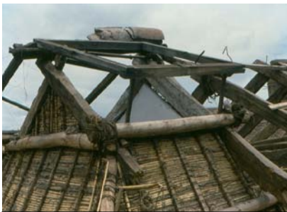
Figure 7: Skylight. Note the wood structure and "chahuarquero" battens. The soffit is supported by a layer of vegetal fiber made of reed or "chacilla".
