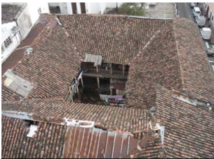
Figures 18: Traditional typology of roof configuration. Note the unity of the architectural system but also factors of deterioration..
