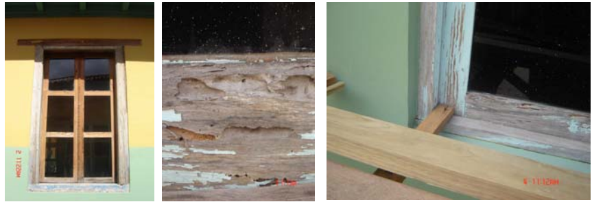
Figure 16: Window frame, termite attack on window element, scaffolding nailed to window frame.
