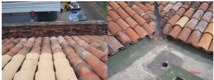
Figure 13: Roof tiles do not match existing ones. Parapet wall is exposed to weathering and lacks capping. Valley canals are zinc made; downspouts in main canal are not protected.
