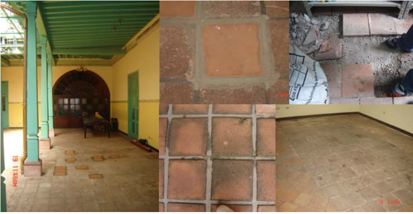
Figure 18: Replaced tiles in corridor outstand because of difference in material. Close up of new terracotta tile and joints. Presence of humidity and mold in tiles. Testimony of original tiles in a room, the quality is superior to those used in later repairs.
