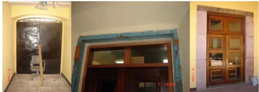
Figure 17: Replaced metal door in basement access. Door frame painting peeling and wooden repaired parts.
