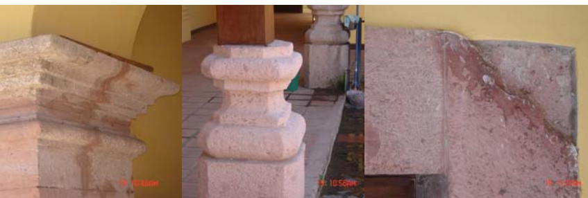
Figure 20: Repaired joint, porous stone and mold growth, repaired door detail.
