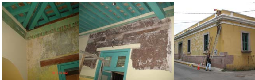
Figure 15: Wall humidity at the bottom of roof canals, untraditional repair with wire mesh, and industrial gypsum compound for repairing cracks in exterior walls, and humidity and mold at unprotected bottom of exterior walls.
