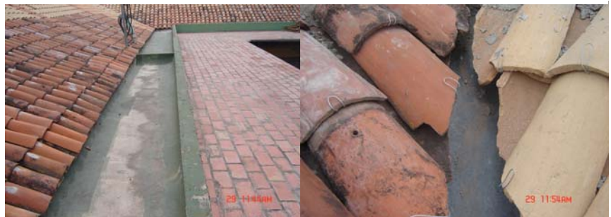
Figure 14: Partitions in main roof canal are due to insufficient slope for water to evacuate. Tile fasted with galvanized wire.
