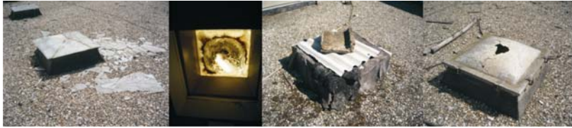
Figure 14. Damaged roof lights
