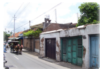
Pictures of buildings damaged by the earthquake 2006
