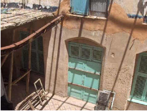
Figure No. 6 Deteriorating conditions
