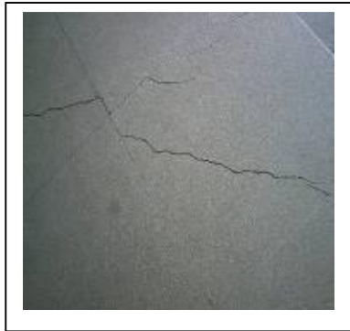
Plate 16: Cracks on the terrazzo floor
