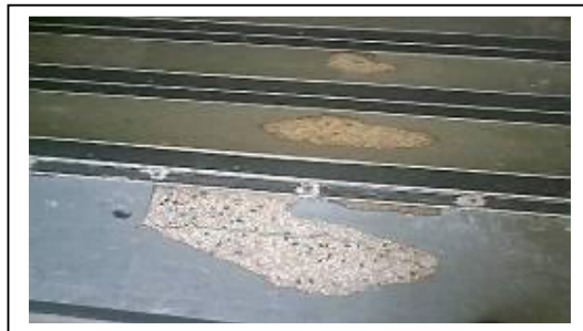
Plate 15: Staircase treads have deteriorated Source: Author, 2009
