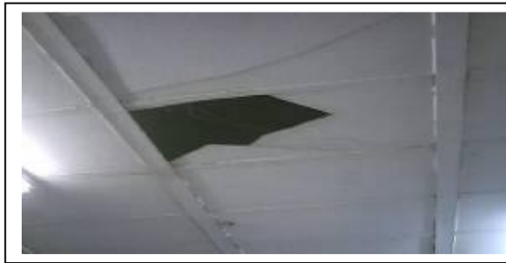
Plate 14: Poor state of ceiling Source: Author, 2009
