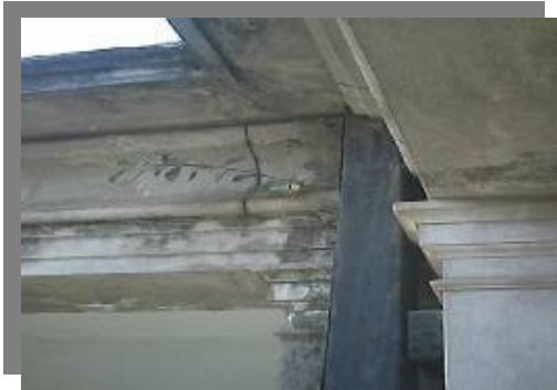
Plate 13: Concrete moulding and blocks have been attacked by plants and algae,
