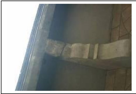
Plate 12: Cracks are due to ground transmitted vehicular vibration
