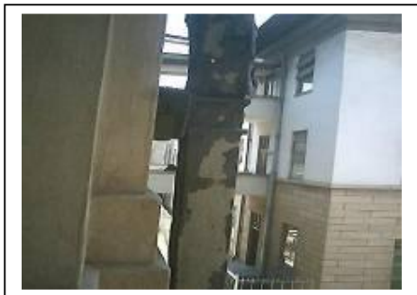
Plate 17: Drain pipe have corroded
