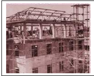
Plate 10: construction process in 1926 ; Steel trusses columns and beams (reinforced concrete). Source: Kenya Railways, 1926
