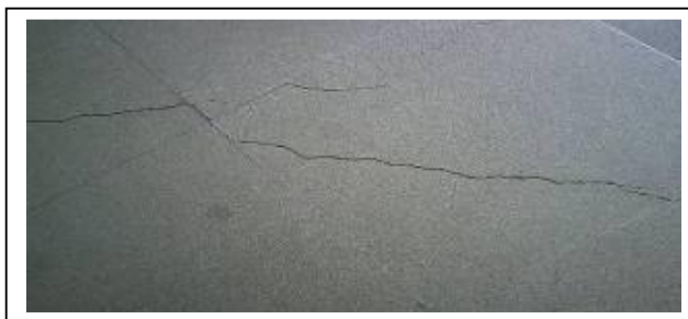
Plate 11: Cracks on the floor are due to ground transmitted vehicular vibration Source: Author, 2009
