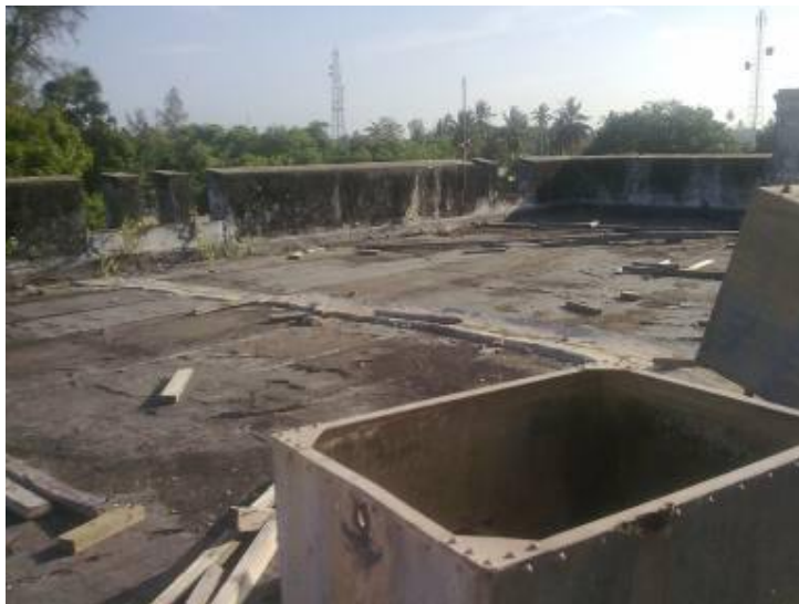
Figure 17: The peeled off of bituminous felt on the roofing slab
