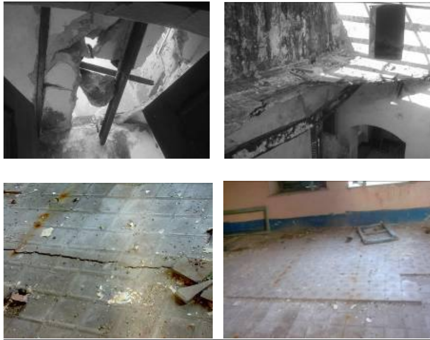
Figure 11-: The poor condition of floor slab and floor finish
