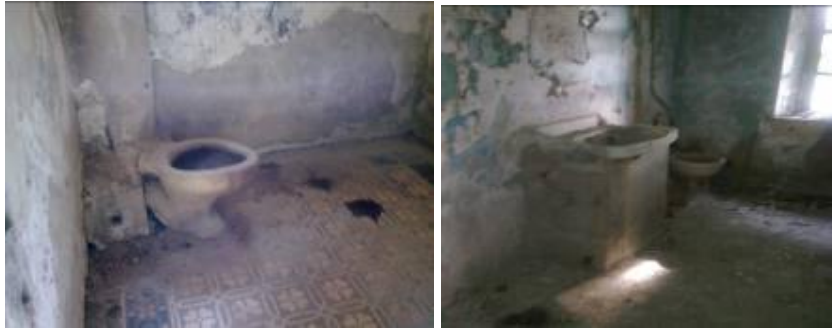
Figure 18: Unused sanitary appliances in very unhygienic condition
