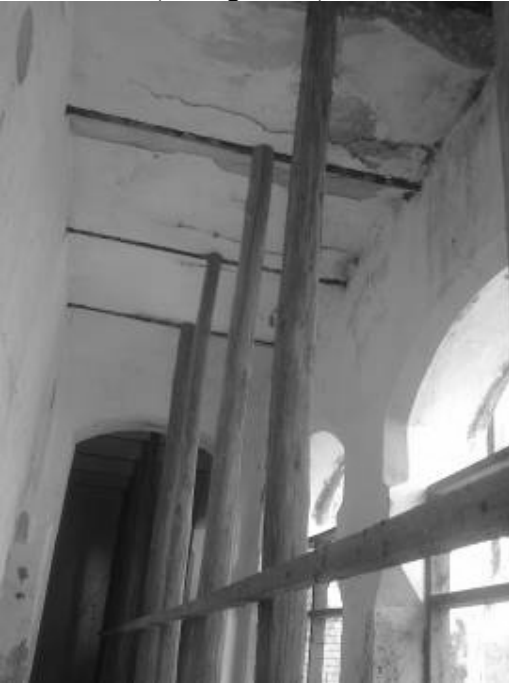
Figure 22: Efforts to protect the building from further deterioration
