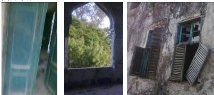
Figure 12 : Absence of window panel, broken windows and flaking painting in existing openings
