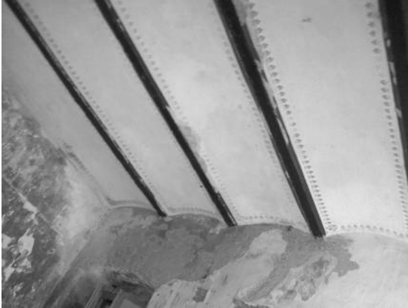
Figure 16 : Poor condition of ceiling vaults
