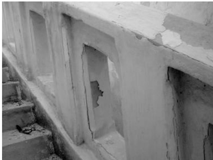
Figure 15: Cracks and mortar peeling off on main staircase balustrades.
