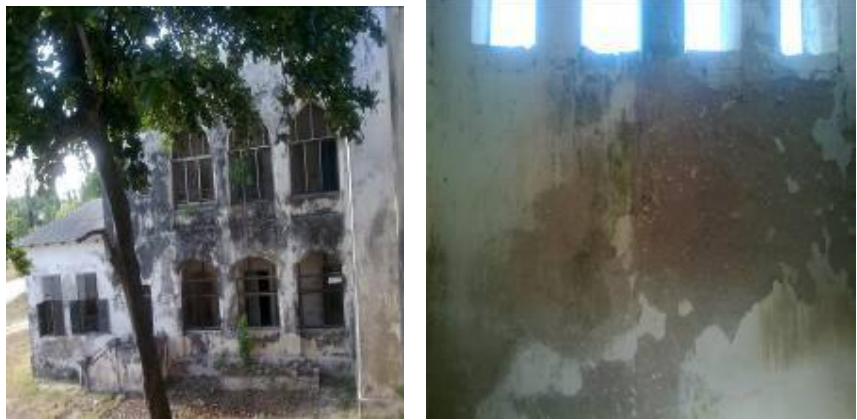
Figure 14: External and internal wall defects
