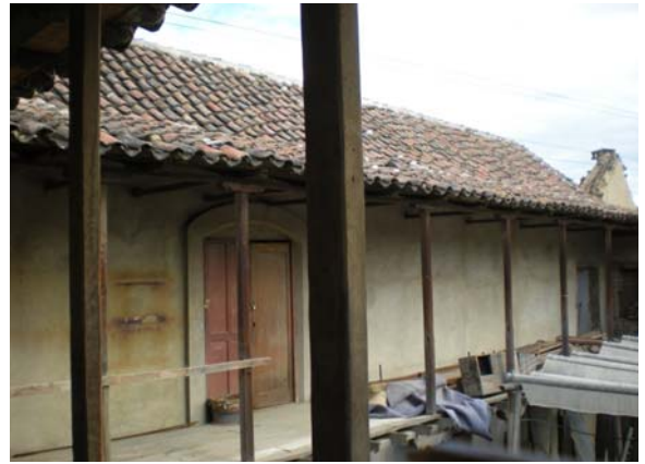
View of the gallerie in the second floor. See the absence of the floor.
