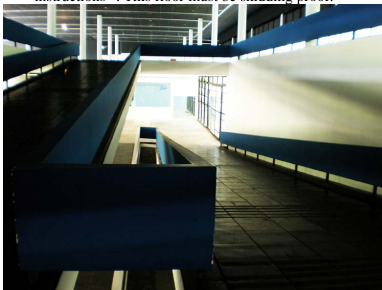
Figure 15: internal ramps with the existing rubber floor ( Plurigoma ) and masonry handrails with iron structure.
