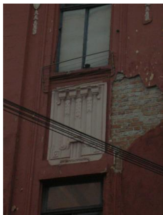
Facade detail showing missing parts of the rendering.
