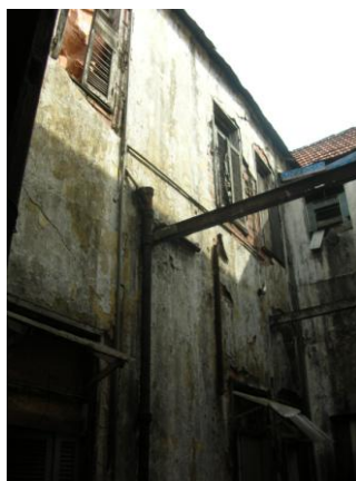
View from the central patio, showing carpentry condition and structural reinforcement.
