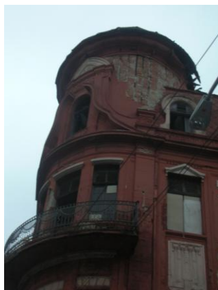
View of the cupola showing missing render on the brick walls.
