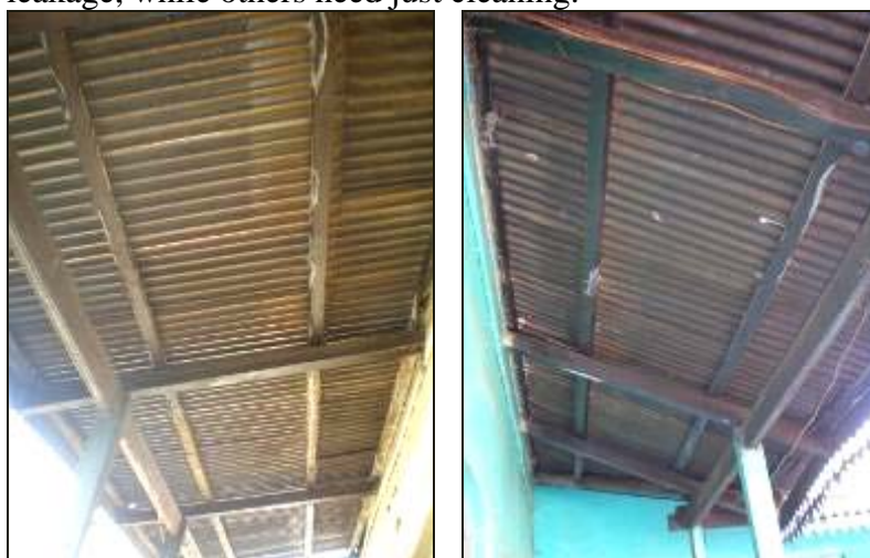
Fig.3.12. Roof top iron sheets are corroded
