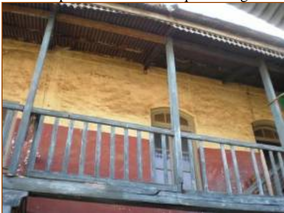
Fig.3.2. Painting done recently which is inappropriate
