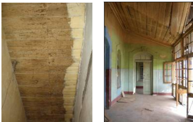
Fig 3.15. Decaying interior space
