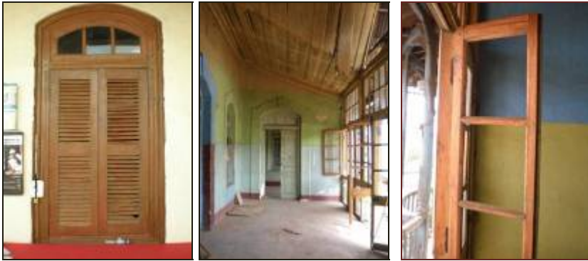
Fig.3.13. Windows are damaged, which needs a lot glazing work
