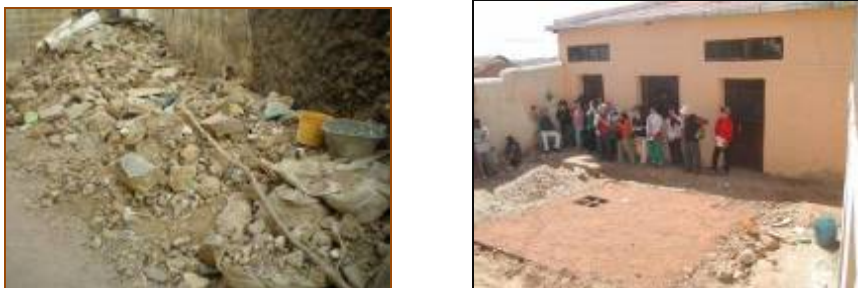
Fig.3.6. Piled up earthing against the building, and inappropriate water reservoir building works in the compound.
