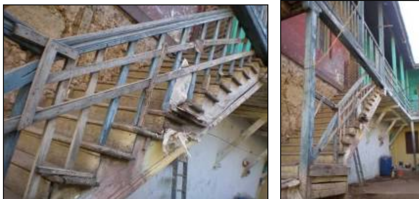
Fig 3.14. Dilapidated stairs to the first floor
