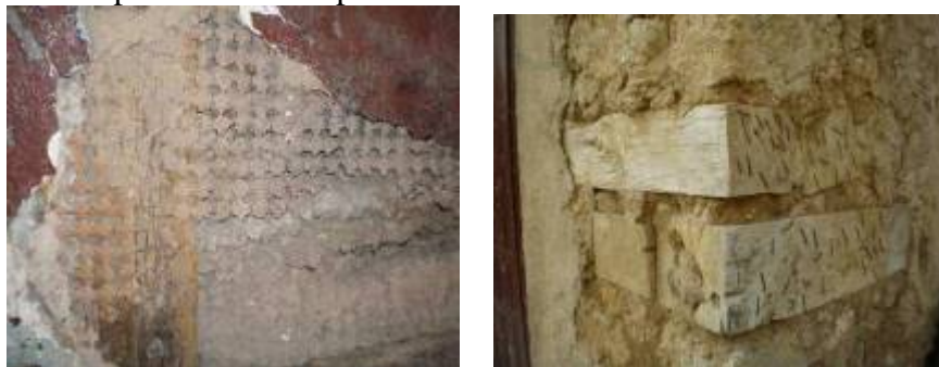
Fig 3.9. damages to the masonry from 1rst floor and ground floor accordingly.
