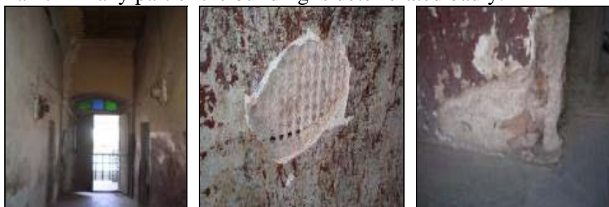
Fig.3.10. Deteriorated paint on different part of the house
