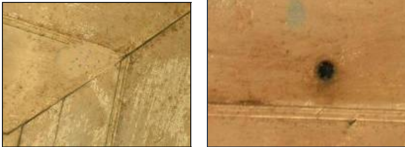
Fig.3.5. Insect infestation on the ceiling of the first floor
