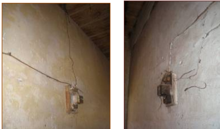
Fig. 3.16. Inappropriate electrical wires
