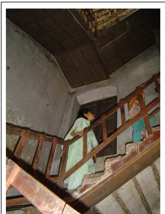
Fig: 18 Vulnerable Wooden Stair
