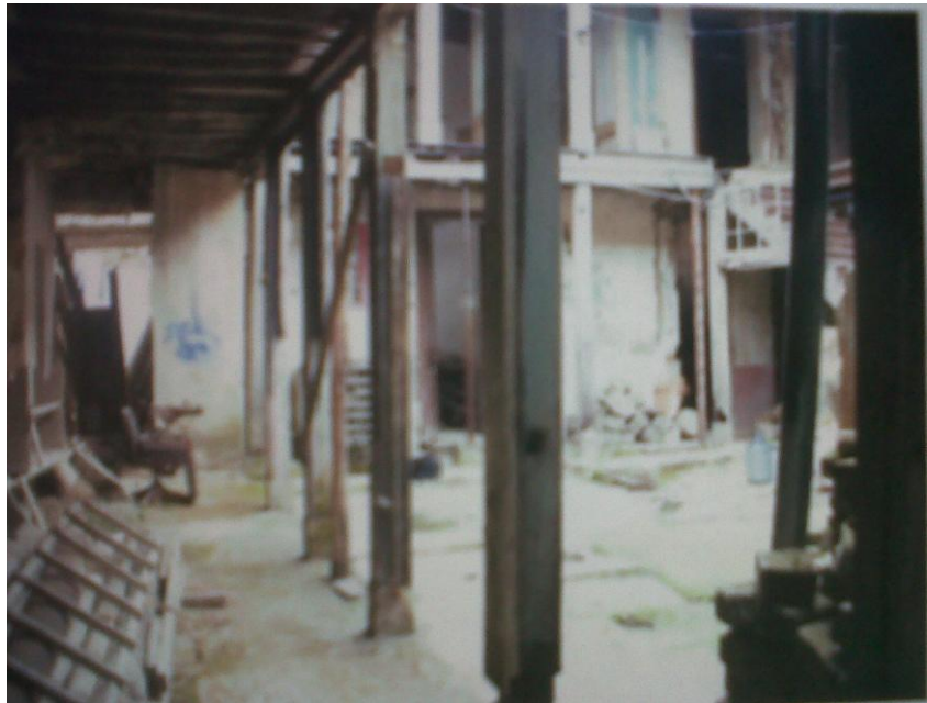
Figure 8: Interior open space, wooden columns have to be replaced or treated to guaranty stability of upper balcony.
