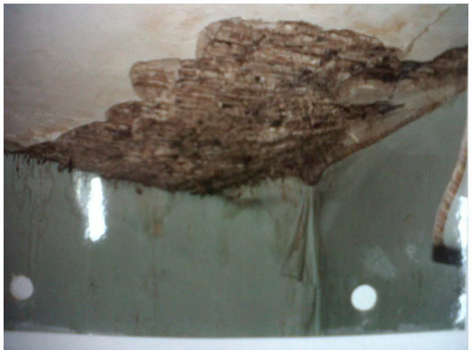
Figure 7: leaks seen on first floor ceiling deteriorating structure.
