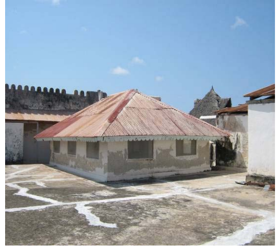
Cracks on the second floor slab.
