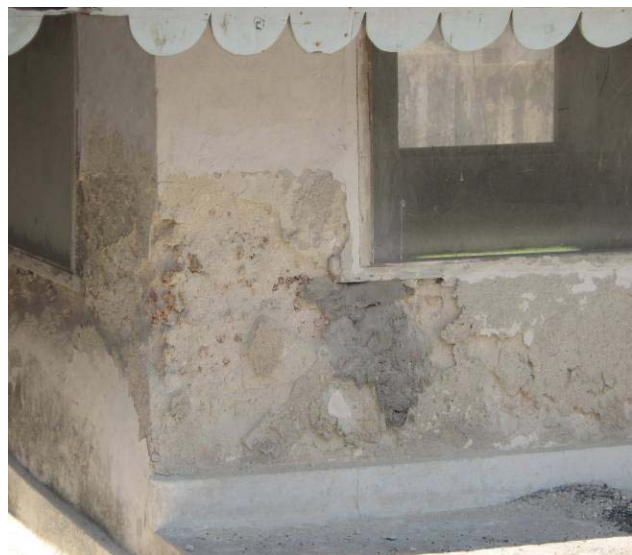
Deteriorated plaster work
