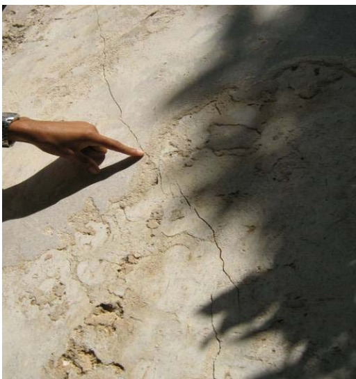
Cracks on wall surface.
