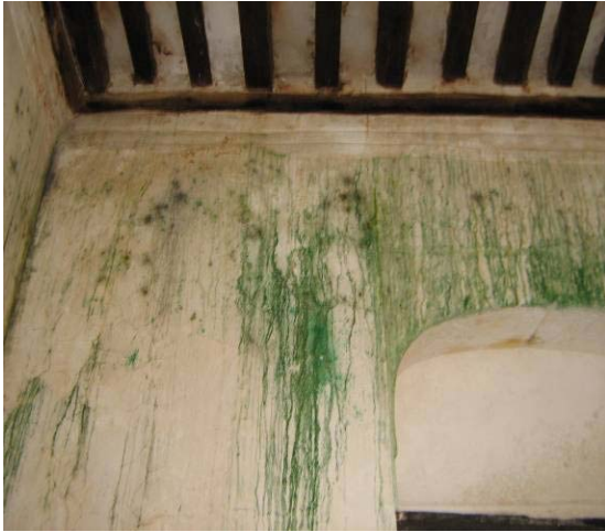
Stained walls due to infiltration.
