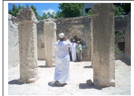
PLATE 7: The mosques traditional roof was seriously dilapidated and had to be reconstructed anew using the traditional techniques and materials
