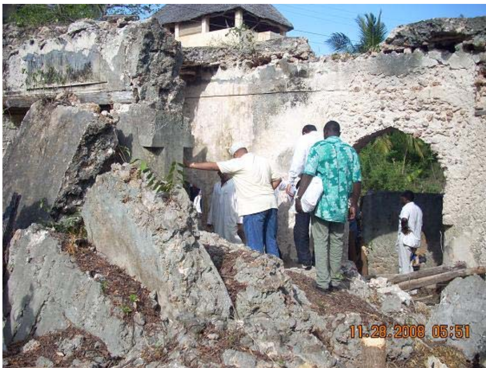
Plate 10 The roof of the mosque had completed collapse and was earmarked for complete reconstruction
