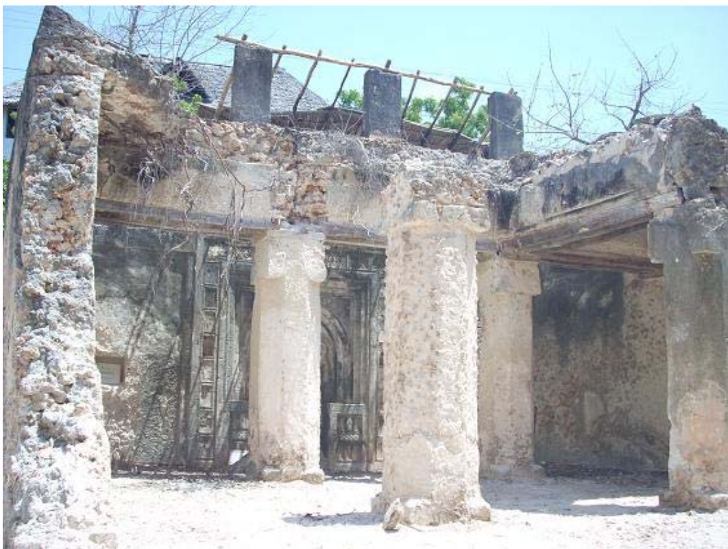
Plate 14. Interior of the mosque .many components of the roof structure had been extensively damaged and needed to be replaced
