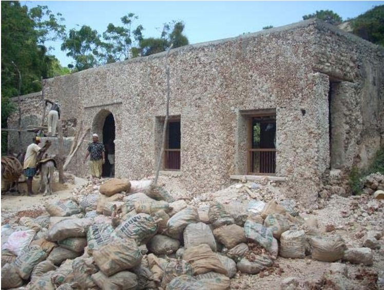
Plate 21: shows the rehabilitated eastern façade .new window openings had to be introduced to improve the air circulation and lighting inside the mosque.
