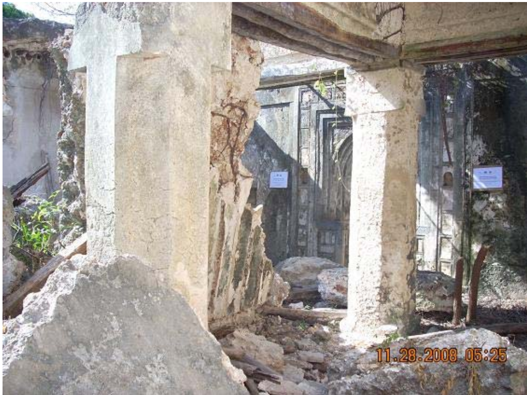
Plate 11. Interior of the mosque before rubble from the collapsed roof was removed
