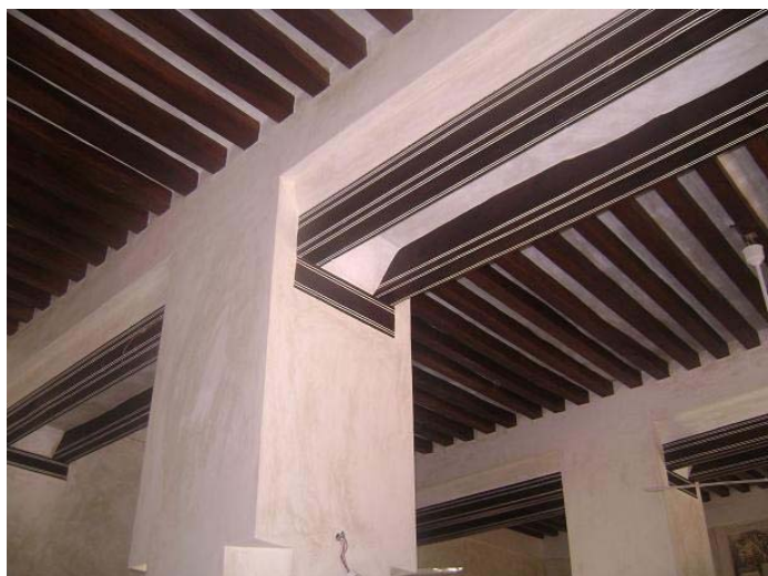
Plate 25.reconstructed roof slab of the mosque.this was the only component to be fully rebuilt.
