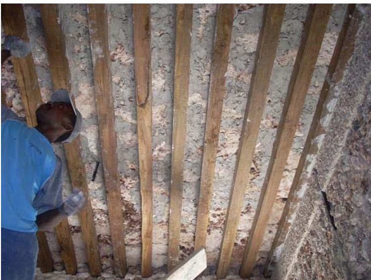
Plate 23. filling the joints of the coral rag bed laid over the timber ceiling joists. this is the traditional technique used in constructing suspended floors in Swahili buildings.
