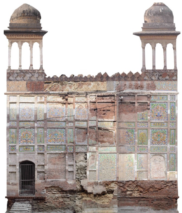
Existing South Elevation of the Gate Way in a Dilapidated Condition
