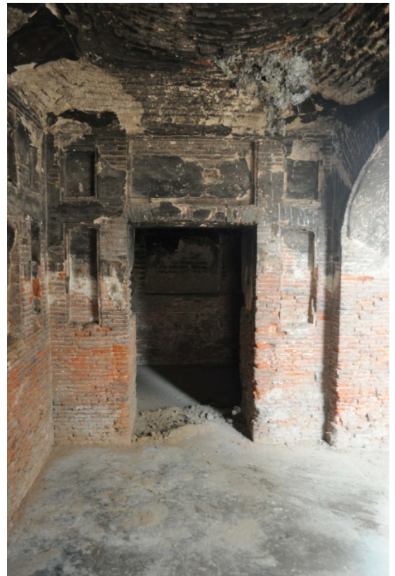
The decorative Ghalib Kari has been completely vanished from ceiling.
