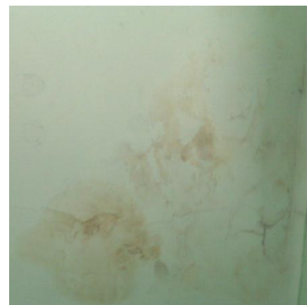
Figure 16: Humidity in walls
