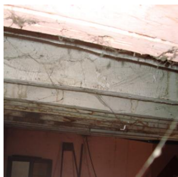
Figure 35: Cobwebs in beams
