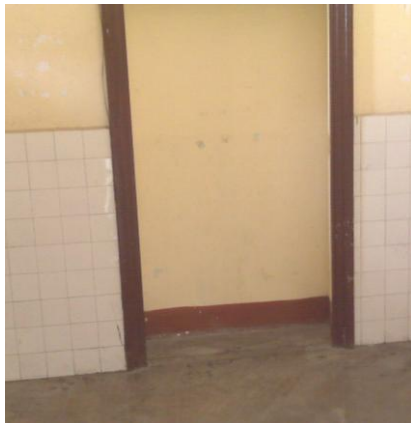
Figure 29: Door closed with a wooden board
