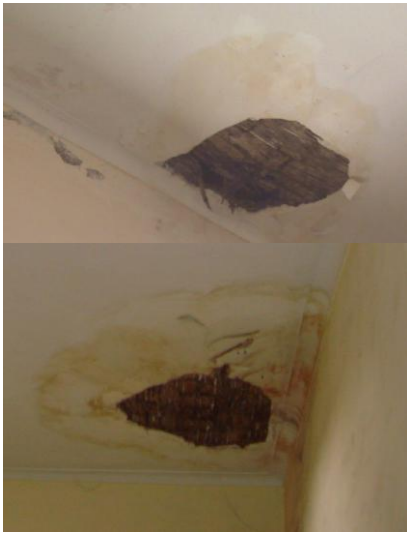
Figure 17: Leaks in quincha roofs
