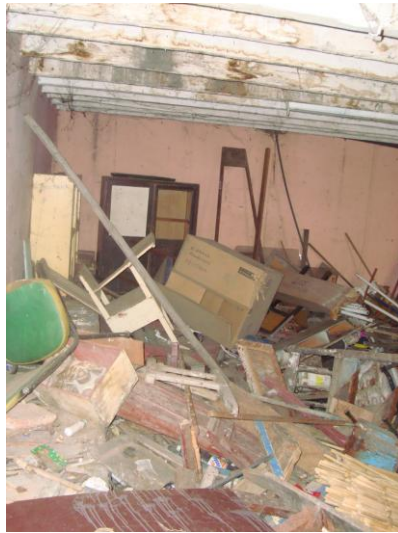
Figure 18 Leaks in quincha roofs
