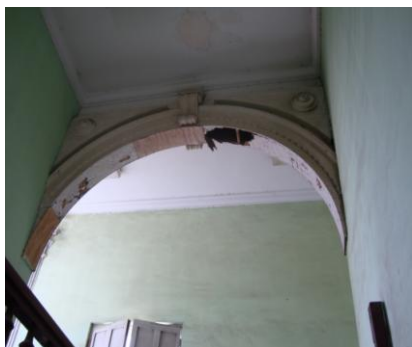
Figure 26: Damaged intrados of wooden arc
