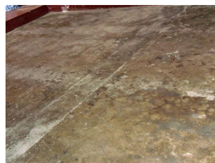
Figure 34: Footprint of an adobe wall removed.
