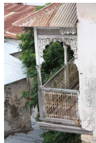
Figure 14 Balcony in bad condition
