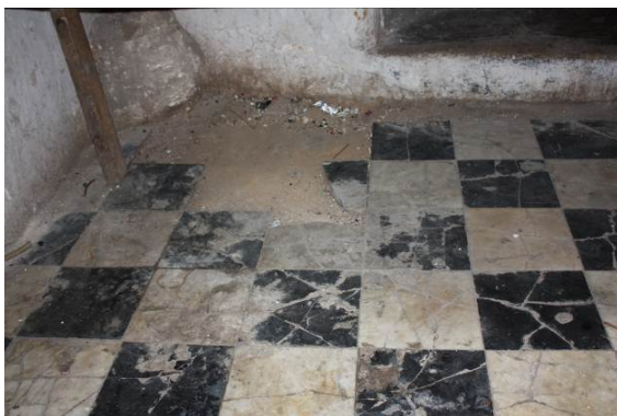
Figure 21 Original marbles in poor condition
