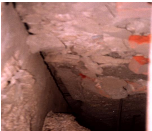
Cracks on roof
