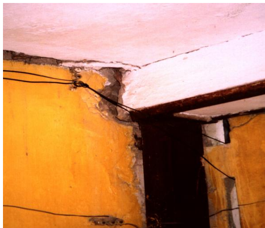
Cracks on beams
