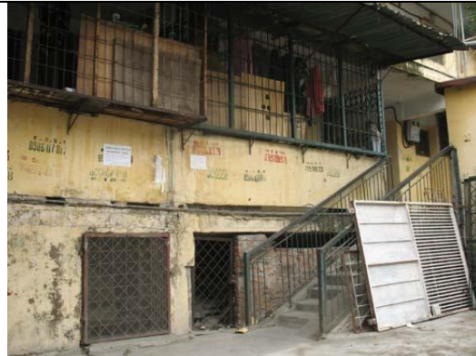
Apartment building C1 in Giang Vo sank 1.5 m and leaned 15 degrees (Vietbao.net 2008/2/28)
