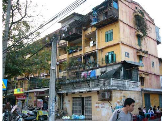
B6 – The dangerous apartment building in Giang Vo (Vietnamnet 2007/2/3)
