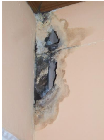
Figure 2: Damaging the water seal on the surface creates water seepage problem
