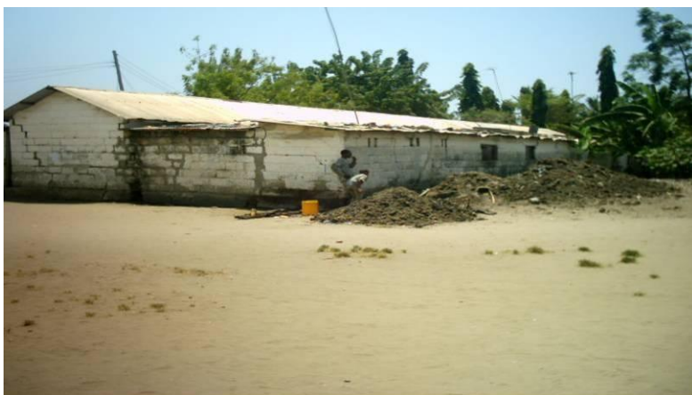
Kawe Mzimuni House with cracks, residents emptying a pit latrine to a nearby external pit.
