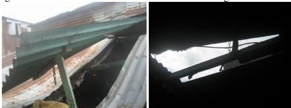
Fig 19 & 20: Temperature is so uncomfortable that they had to open the ceiling.
