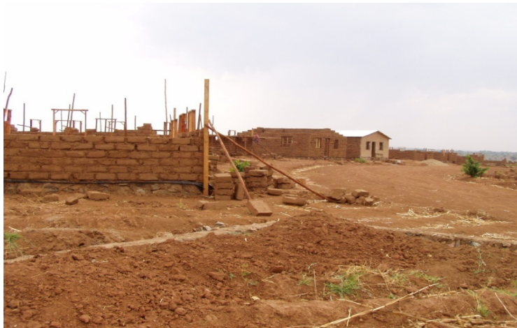
Figure 3 : Low income houses under construction supported by CCODE on land provided and serviced by Lilongwe City Assembly in Area 49
