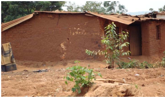
Figure 6: Poor Quality Housing in Mchesi Informal Settlement in Lilongwe
