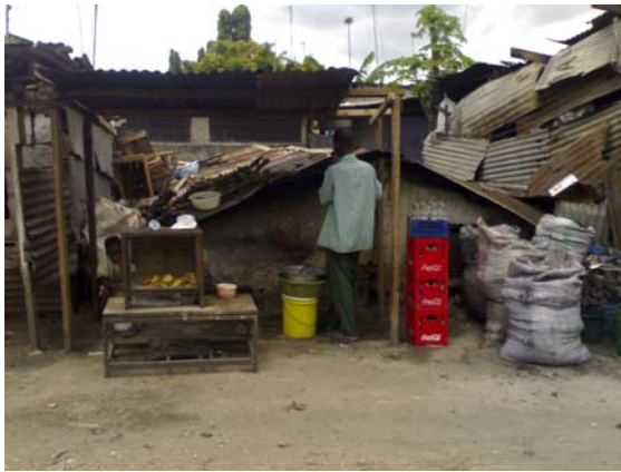
Poor design, workmanship & low technology in building construction
