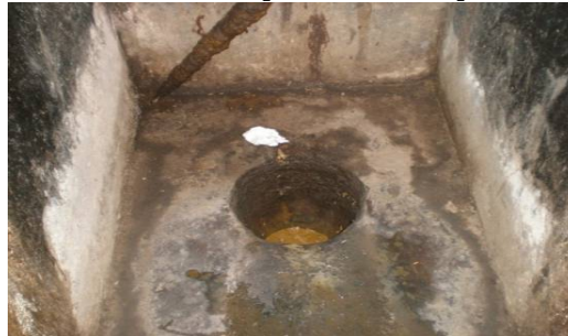
Plate 7: A Communal pit latrine in a deplorable state
