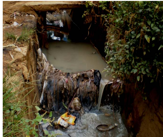
Picture 3: Poor drainage as seen in Katanga – kannala
