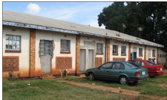
Fig. 5.0 A Metal workshop converted into living Quarters due to critical housing shortage at David Kaunda Technical High School in Lusaka District. Picture by Author, January 2010
