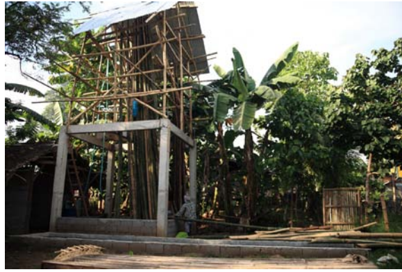
Figure 6 VSD treatment plant in Matina community
