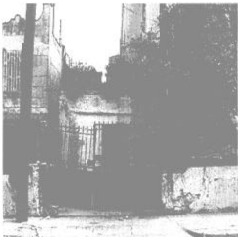
Figure 2. Lack of maintenance and housing deterioration.
