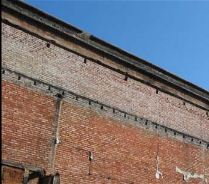
Photo N° 3: Fire wall building leaned by street Santiago Severín.
