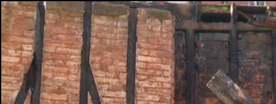
Foto N° 8: Image of present state of tabiquería interior of wood with bricklaying of bricks. Image of present state of tabiquería interior of wood with bricklaying of bricks
