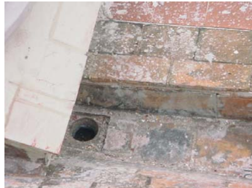
figure 60: Loss of gratings
