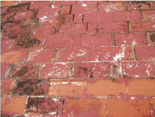
figure 44: Tiles broken and loss of joint material
