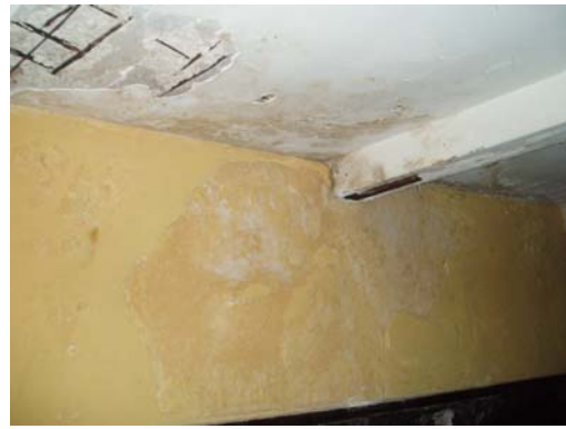
figure 46: Interior walls - Moisture surfaces
