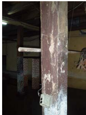
figure 47: Structure affected by termites
