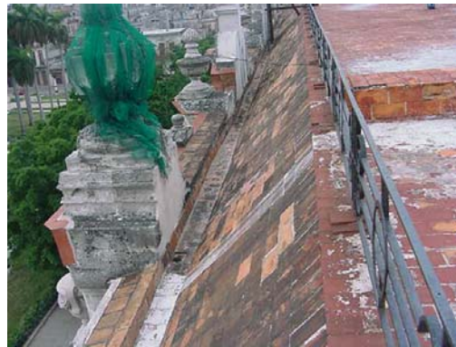
figure 64: Damaged elements on the roof
