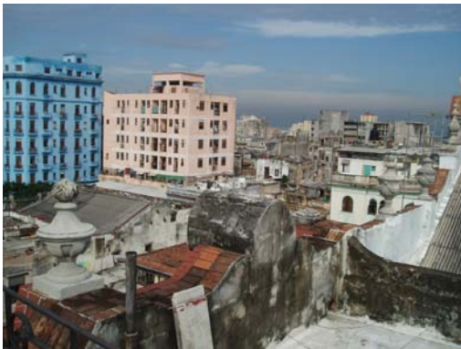
figure 63: Damaged elements on the roof
