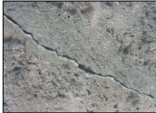
figure 52: Rupture- Prado facade
