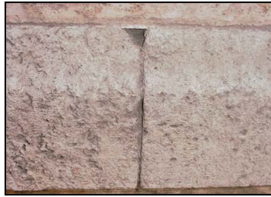
figure 50: Loss of joint material.-San Jose facade
