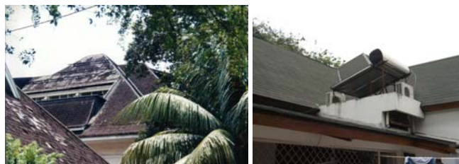
Picture 13: The old and new roof cover material, shingled roof removed to fiber-concrete.
