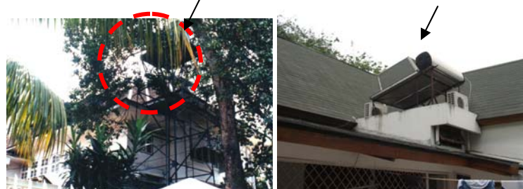
Picture 17: The old water tower at front side and the hidden equipment at back side.
