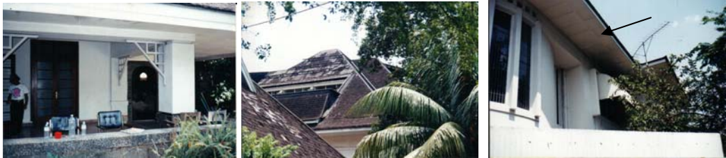
Picture 10: Bearing wall structure, roof material and the damage of ceiling caused of leakage.
