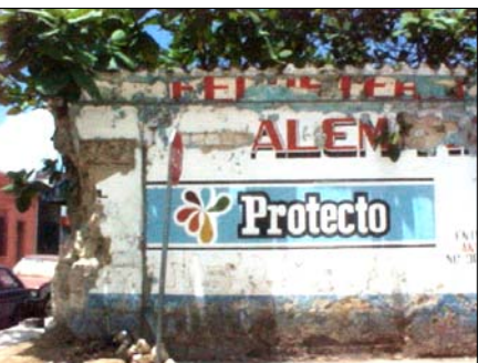
The building conserves only its wall of facade, the interior is covered with vegetation. The facade shows publicity signs. We can see adobe in some sections of the cave in on the corner wall.
