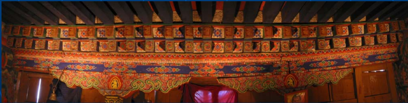
Critical structural members threatening imminent collapse
