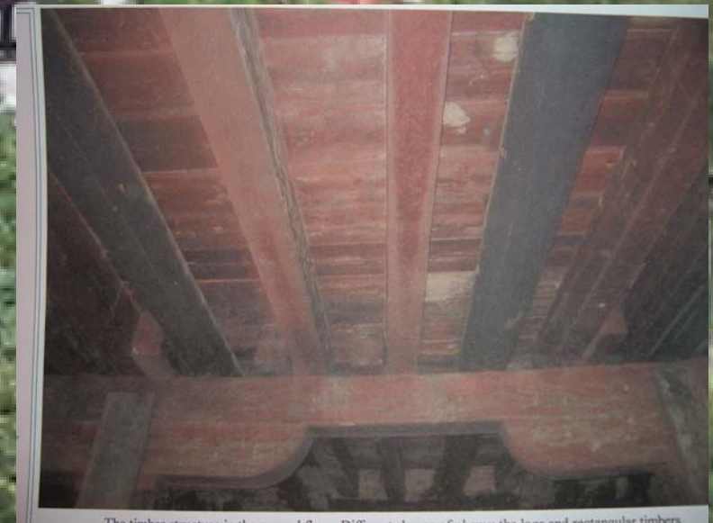
The timber floor structure showing the multi-layered timber slabs and supporting timber beams.
