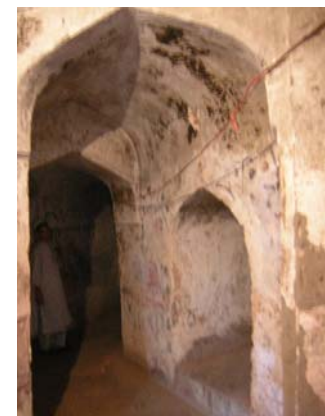
Fig. 29 Damp on wall
