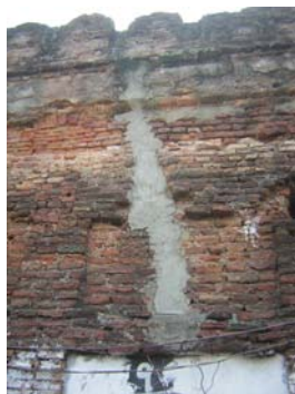
Fig. 22 Major crack on wall
