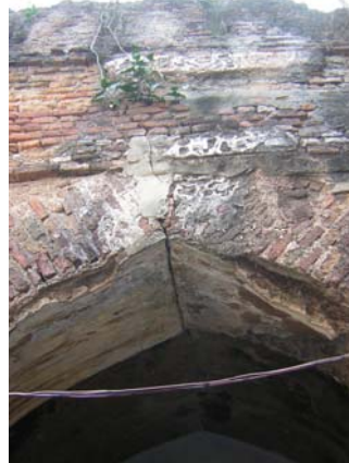
Fig. 28 Crack on arch
