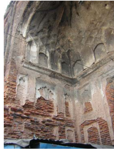
Fig. 44 Damage of plaster detail
