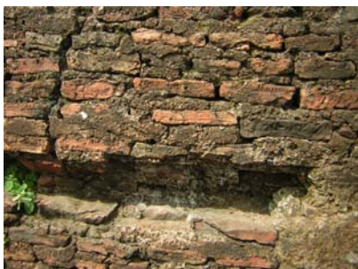
Fig. 33 cracks on wall caused by plant roots
