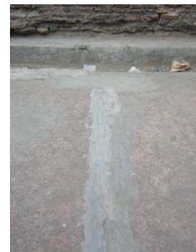
Fig. 24 Continuation of The major crack on floor
