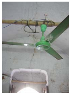
Fig. 23 Continuation of the major crack inside.
