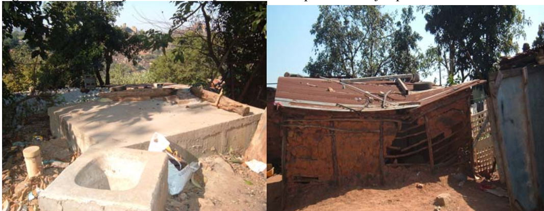
Figure 11 Toilet platform and one of the houses in poor state of repair
