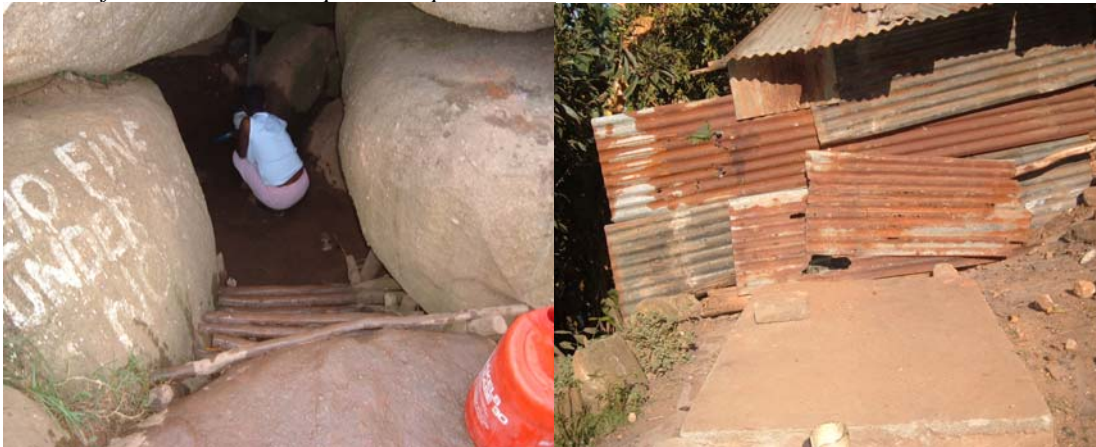
Figure 7 Maqobolwane water collection point surrounded by boulders located right in the middle of the settlement. Uphill are pit latrines like this one next to it
